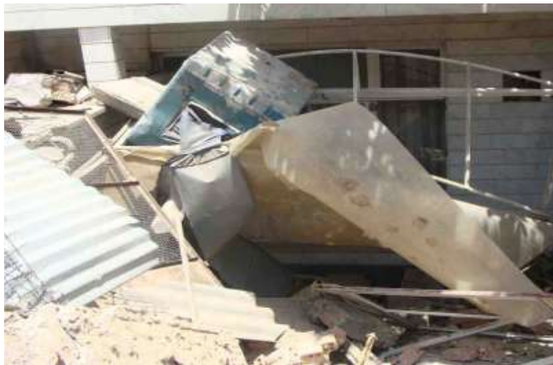
Picture No.16: View of a rubble accident in district 10
