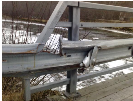
Damaged safety fences
