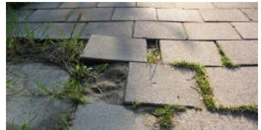
An accident waiting to happen
