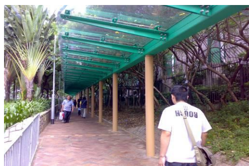
Construction of a covered walkway between Tai Po Market MTR Station and Tai Po Market, Tai Po
